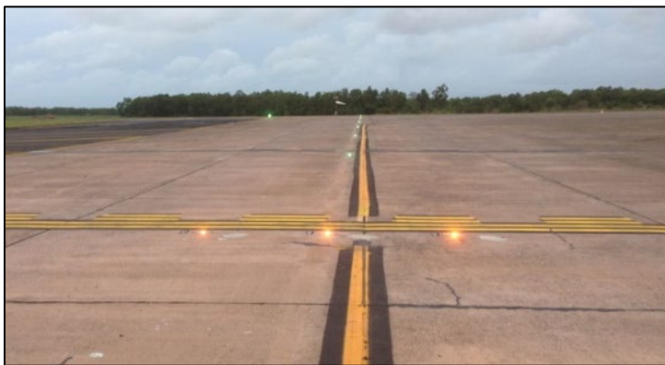
RWY Holding Position Lights
